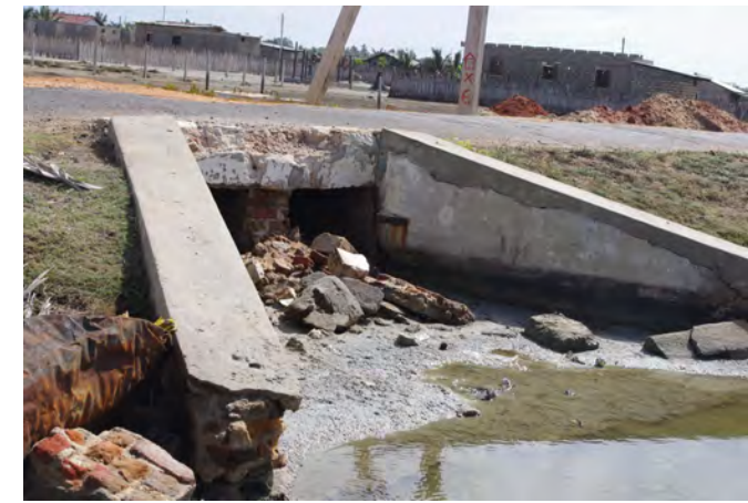
Blocked drainage under Station Road
